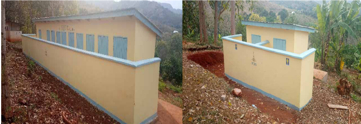
Improved ventilated pit latrines at Diovuva Primary School
