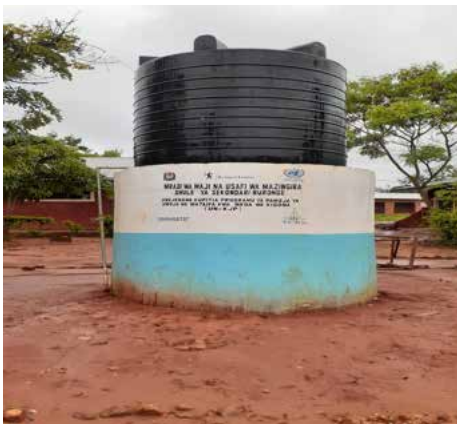
Installed storage tank at Bulonge Secondary School
